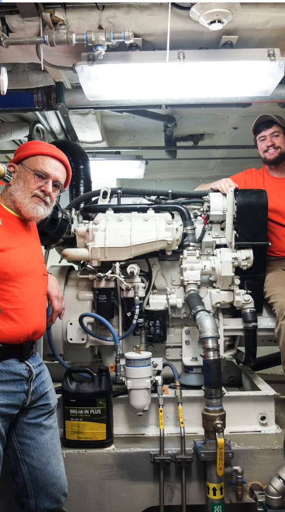
Chief Engineer Dan Luglio (right), and First Engineer Doug Faunt share the importance of the Deere Power Tech 4045AFM85 marine engine equipped with the Logan Front of Engine Power Take-off (PTO) Clutch. Dan is sitting atop the Logan PTO and bracket mounted to the front of the engine.
