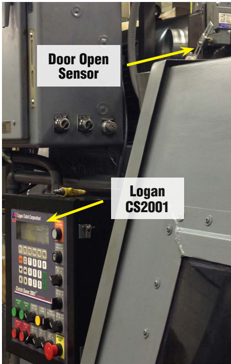
Above: Acme screw machine with Logan CS2001 and Door Interlock Switches (Square D#9007C54B2)
